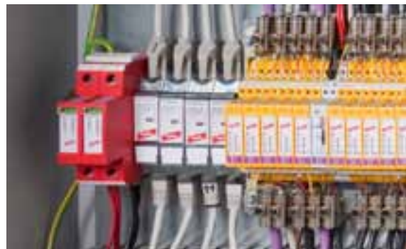
Figure 11 Example of surge protective devices in a pitch system
