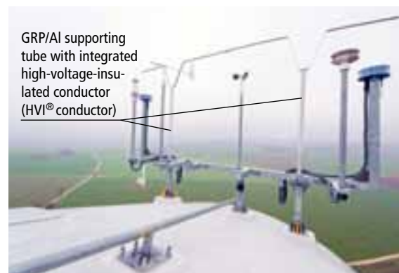
Figure 2 Example of an air-termination system for the weather station (anemometer) and the aircraft warning light
